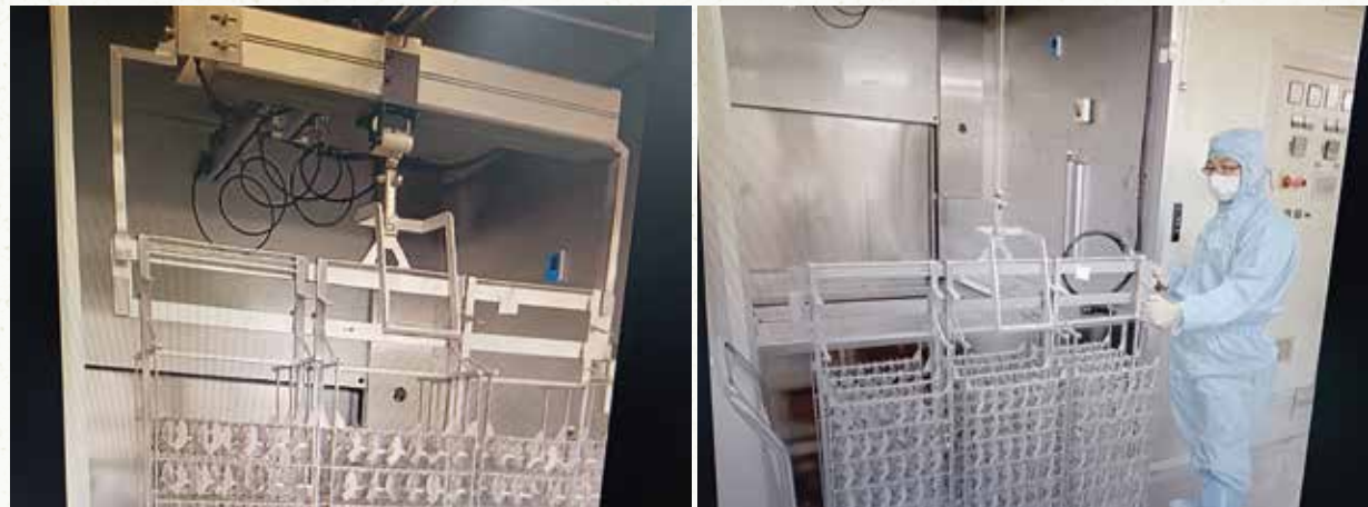
Newly installed Labor-Saving Device
