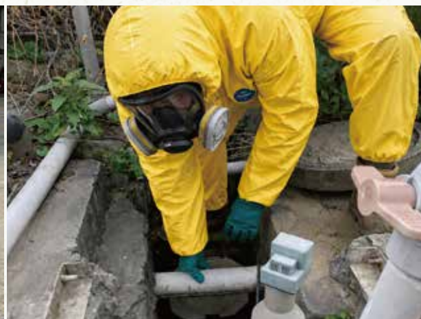
Closing the Stormwater Sluice Gate
